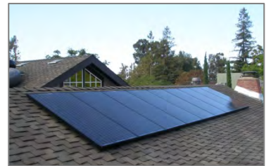
Figure 3.2 Building-mounted solar energy system
