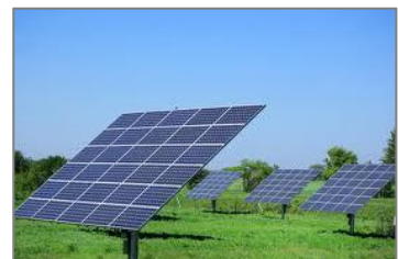
Figure 3.1 Ground-mounted solar energy system.
