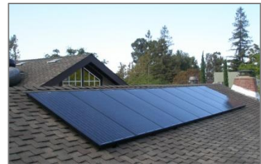
Figure 3.2 Building-mounted solar energy system
